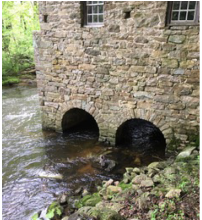
The mill's double-arch outlet is a vital structural component of the building.
